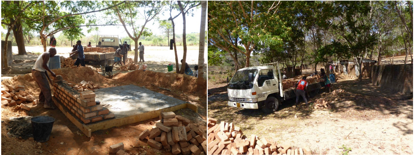
The vehicle being used to transport bricks to Matete Primary School for the construction of a menstrual toilet block there
