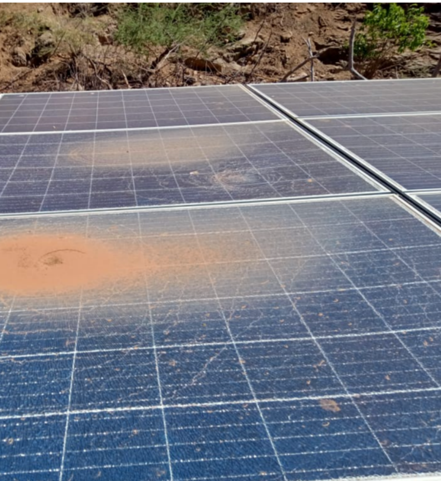
The broken panels
