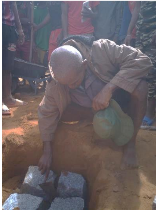
Figure 6 Foundation ceremony : Elder of the village symbolically laying the first stones to the building.
