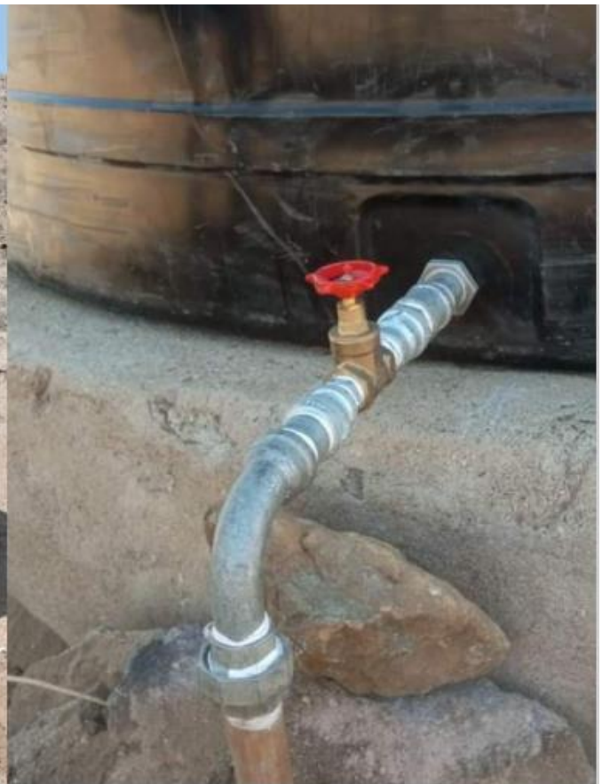
New galvanized pipes and gate valve
