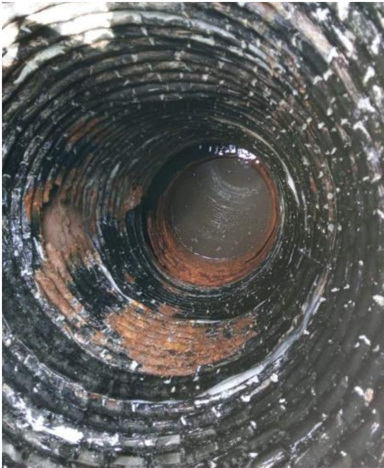
Corroded well lining
