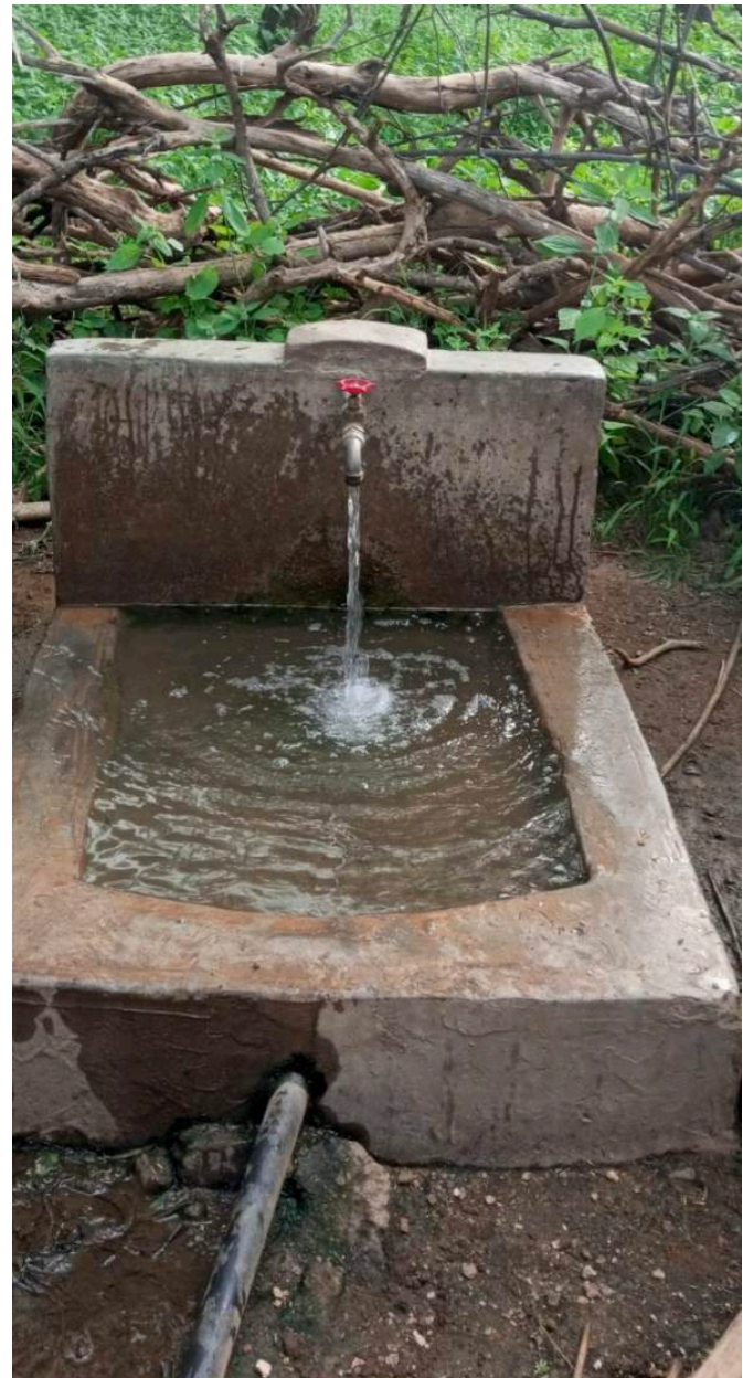
One of the standpipes to be mended, new taps and some leaks to fix
