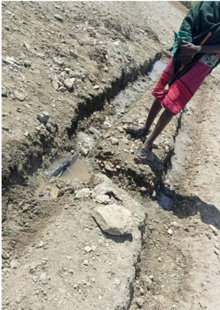
One of the damaged sections
