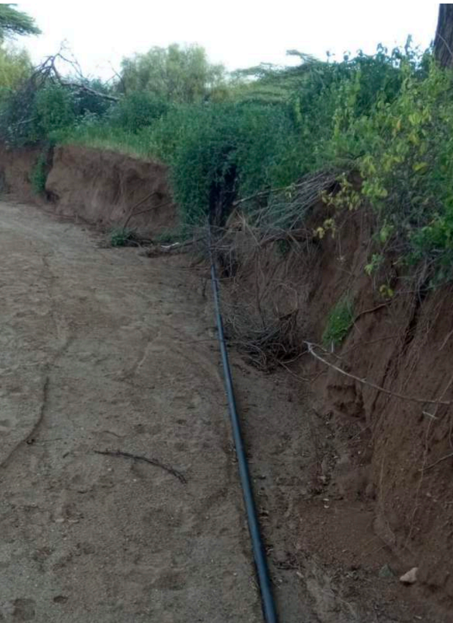
Pipeline washed away
