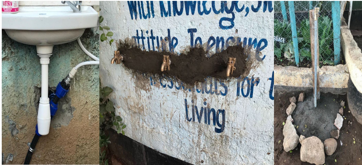
Wash basin, community water access taps and a stand at JM Goodhope School
