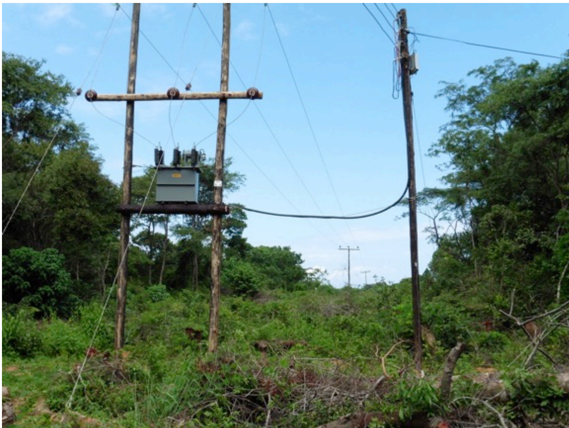
The new transformer in place
