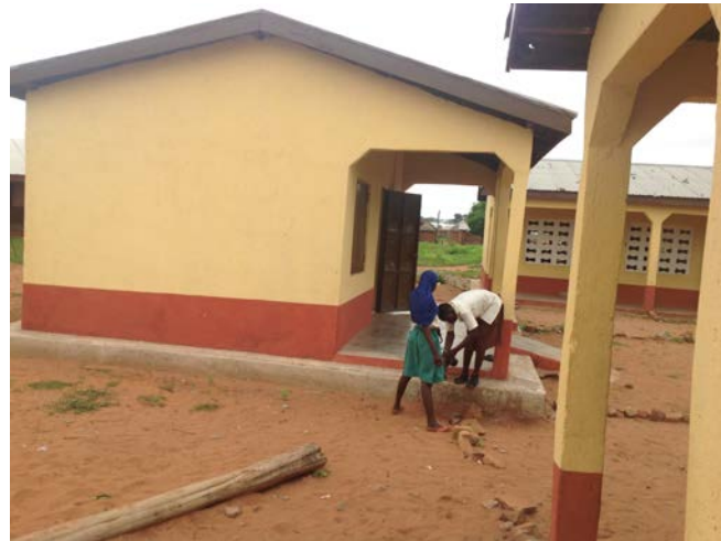
Repaired and repainted Nasyria Primary School showing the aprons, steel doors and newly painted walls of the three blocks, the teacher's storeroom being in the foreground.
