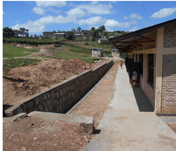
Fig. 2 The wheelchair access can be clearly seen in this photograph, alongside the retaining wall.
