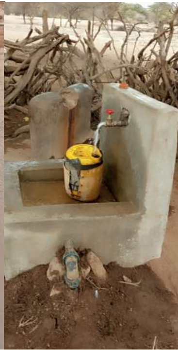
New Community standpipe
