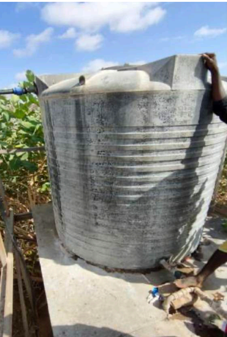
The old tank, damaged by the sun and leaking
