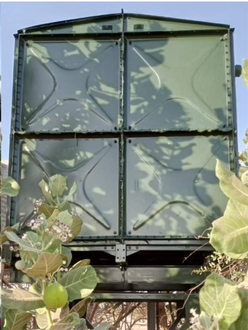
The new steel tank- painted and installed
