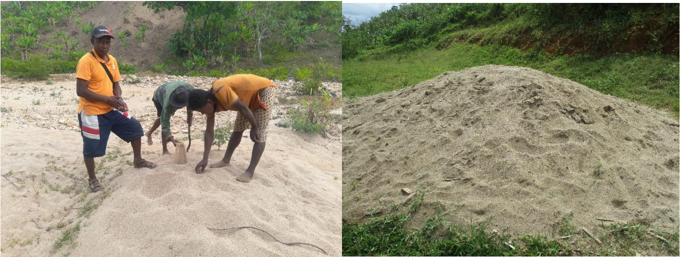
Checking the quality of sand available at source (left) & (right) sand transported to Maromby.
