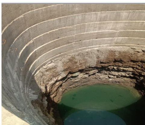
Depth of the well is 50 feet. There is a good amount of water in the well
